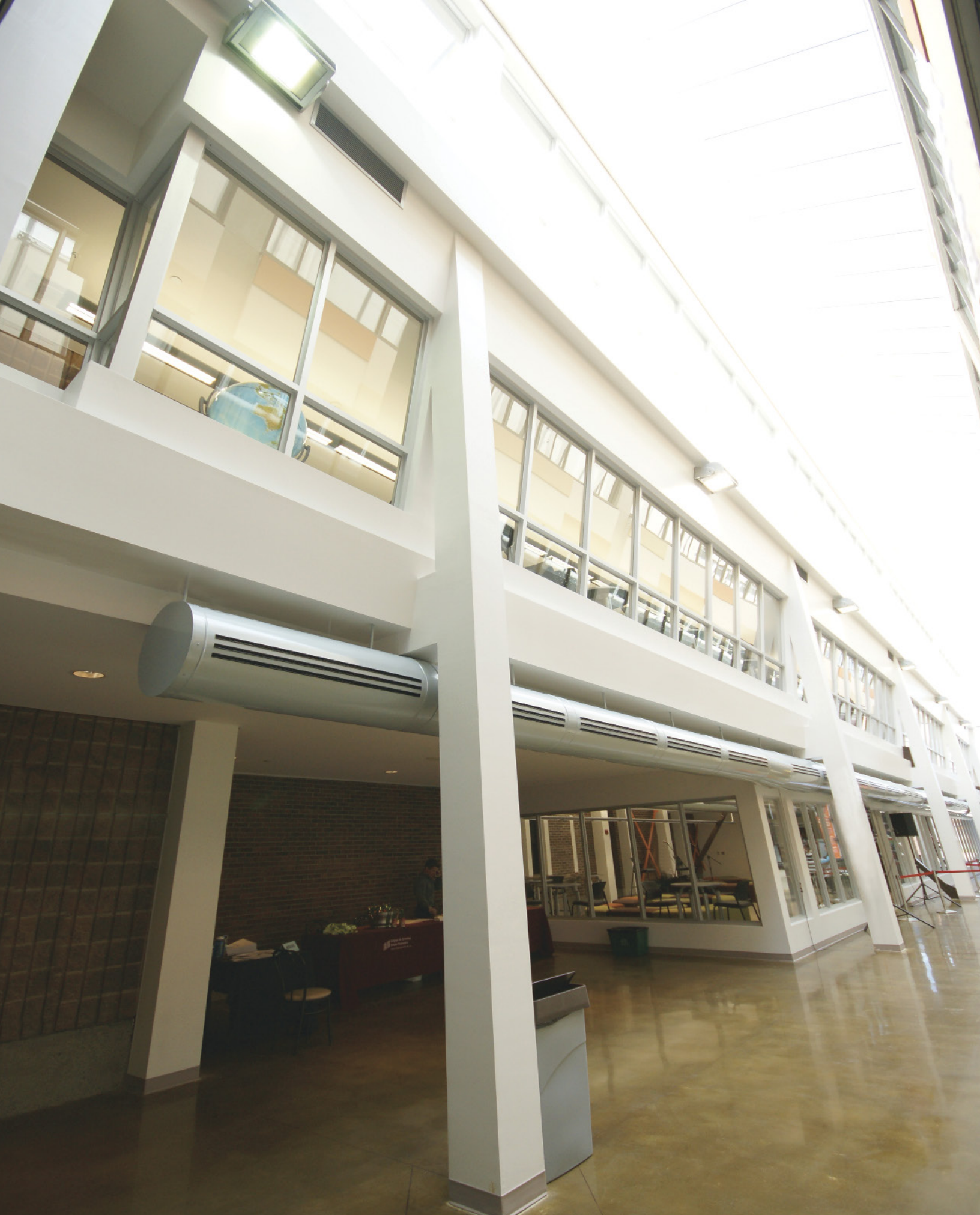
RRA Duct diffuser, Cegep of Granby, Granby, Canada
