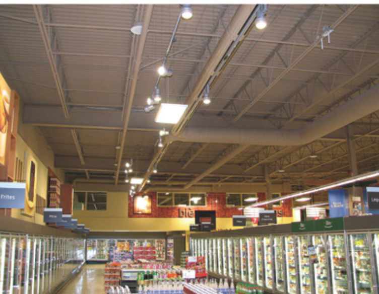
RRA Duct diffusers
