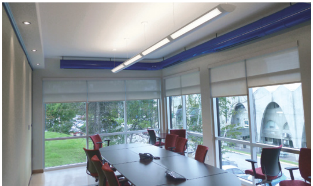
RRA Duct diffuser
